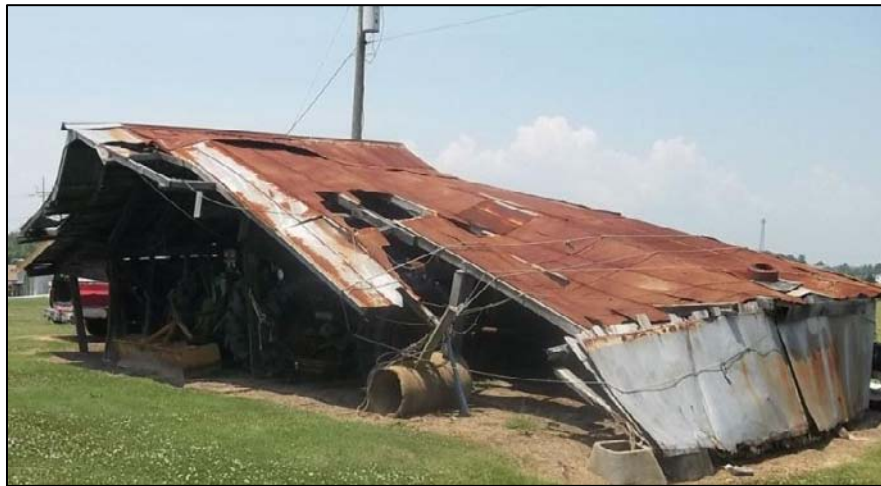
Photo 70: Southeast Oblique of the Dilapidated Outbuilding.
